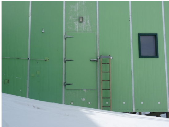
Fire safety is compromised
